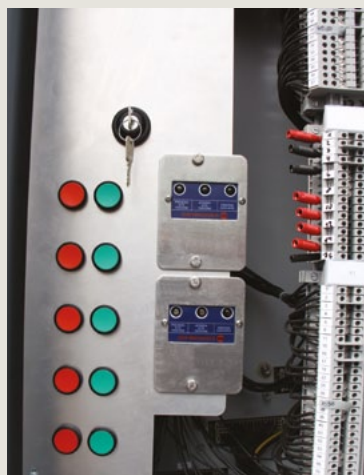
Control cabinet units for the monitoring
