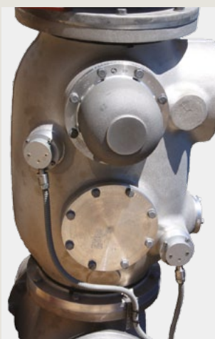
Fixed mounted cameras on the disconnector and earthing switch module
